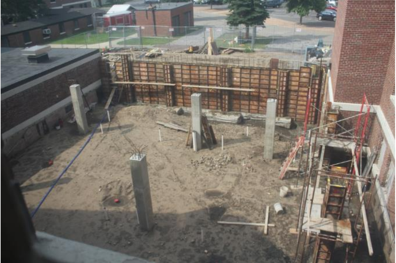
The new Optometry Clinic site at the St. Cloud VA Medical Center now has an exterior wall formed and poured and piers in place. The "infill" of the north side of Bldg. 29 will create an additional 3,800 square feet of state-of-the-art clinical space to accommodate the growing need for optometry services.
