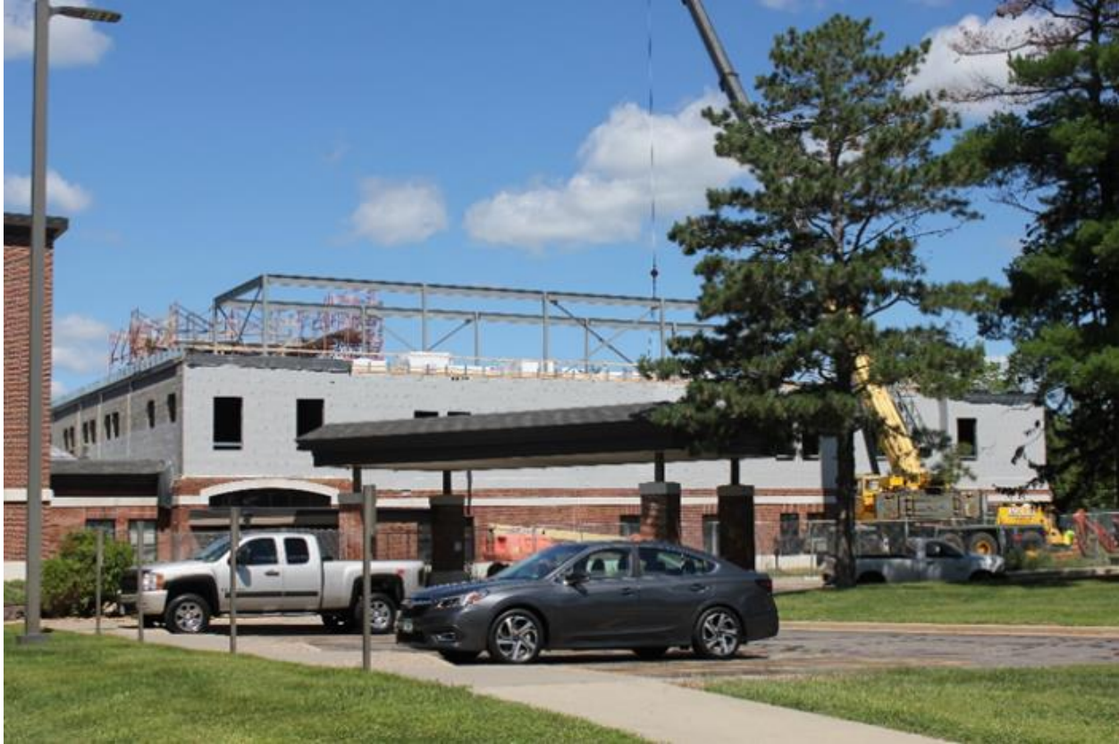
The Mental Health Outpatient Clinic (Bldg. 111) at the St. Cloud VA Medical Center now has the second floor bricked in and the attic is being framed. The additional second floor will create 26 additional counseling rooms and expanded group rooms. The Mental Health Outpatient Clinic is open during construction.
